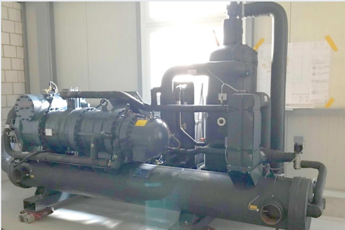
Fig. 1: High temperature heat pump installed at the technical room of the mountain cheese factory [4]. The mildly flammable refrigerant R1234ze(E) demands special measures for fire protection and escape routes.
