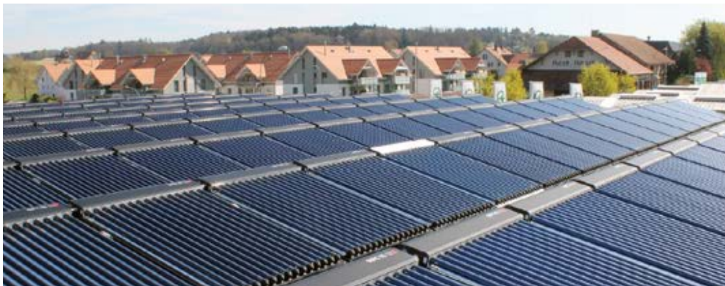
Evacuated tube collectors provide heat for the network of WLS in Schüpfen CH.
