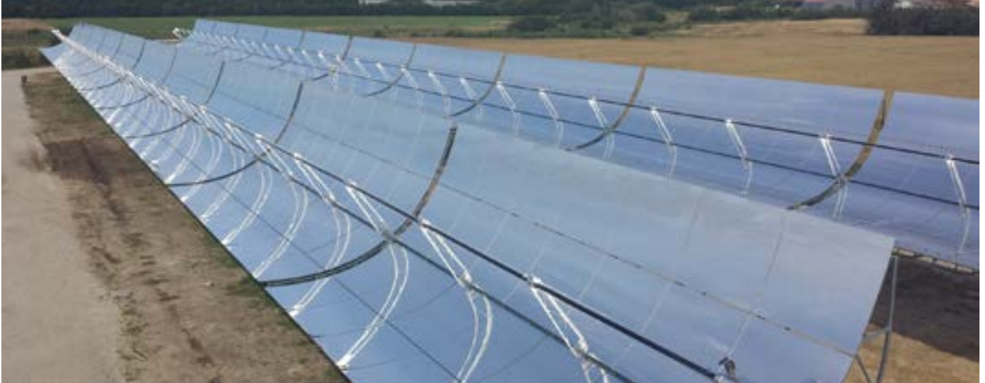
Two collector rows of the parabolic trough collector field in Brønderslev, DK. The 16.6MW t -Plant has an aperture area of 29'929 m 2 and is combined with a biomass-organic rankine cycle for combined heat and power generation. Foto: Brønderslev Forsyning.
