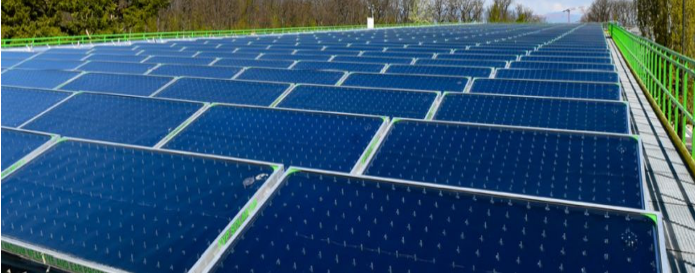
Vacuum flat plate collectors provide heat for the district heating network of Geneva. Source: TVP Solar
