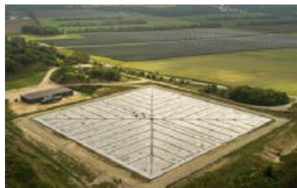
Pit thermal energy storage of Dronninglund (DK), the large solar thermal field installation can be seen in the background. Source: Solites
