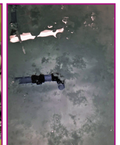
Ice slurry stored with high mass fraction avoiding ice particles from being sucked into the supercooler.
