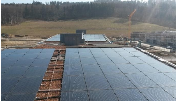
Figure 27: PVT collectors on building C.
