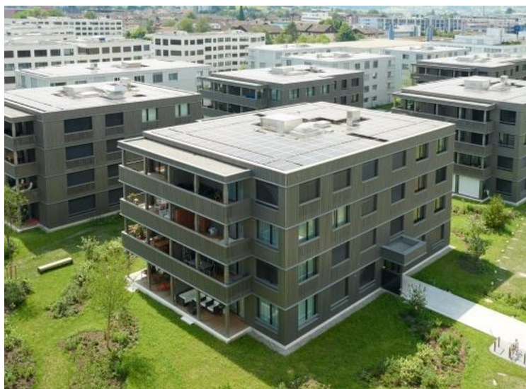
Figure 34: PVT collectors installed on some of the apartment houses in zone 3 of the “Suurstoffi” development site in Rotkreuz. Photo: Zug Estates AG
