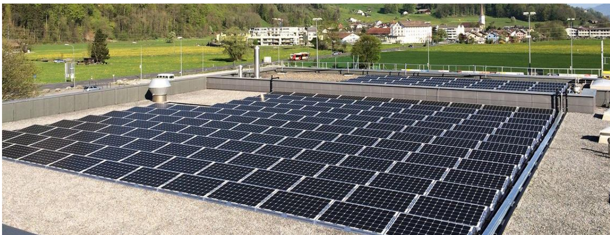
Figure 37: PVT system (292 m 2 ) on the roof of linth-arena. Source: Zurich University of Applied Sciences, Wädenswil.
