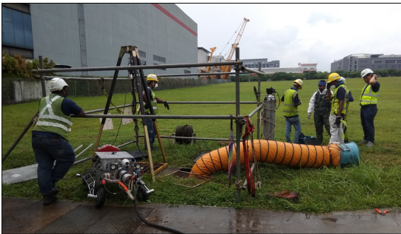
Inspection Robot in front of the sewer access Wei Chuan Law, Robotic Research Centre, NTU, Singapore
